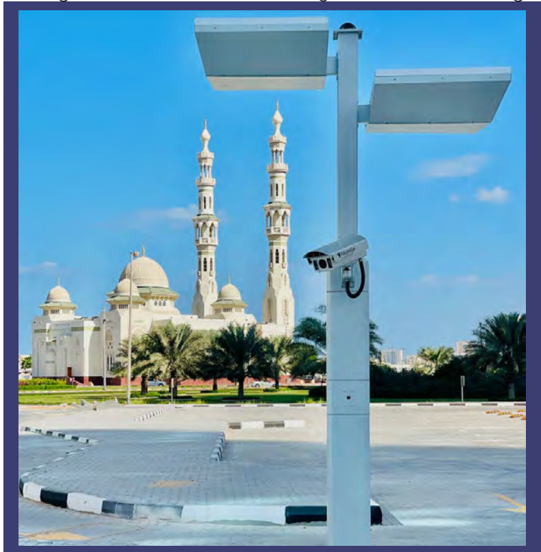
One of the 87 SMART parking poles installed by EIC in Sharjah, UAE.
