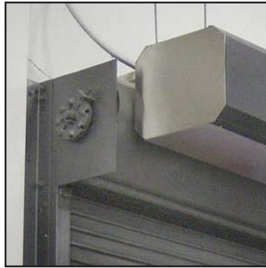
This air curtain is suspended via threaded rod from a high ceiling to hang in front of the canister of a steel roll-up service door.
