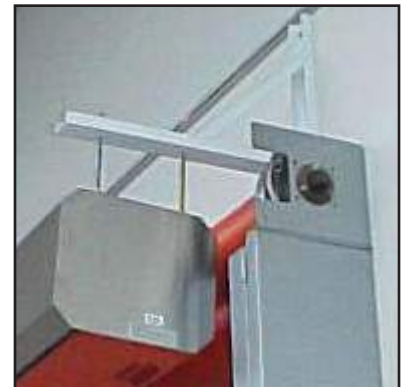
A combination of angle brackets and threaded rod (by others) suspends this air curtain in front of a high-speed roll-up door.
