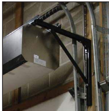
Inverted angle brackets and unistrut facilitate installation outside of door track system.
